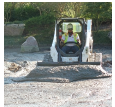
After the koi were safely moved to a temporary pool, crews removed an average of 18 inches of muck accumulated over 24 years from the bottom of the drained ponds and streams.
